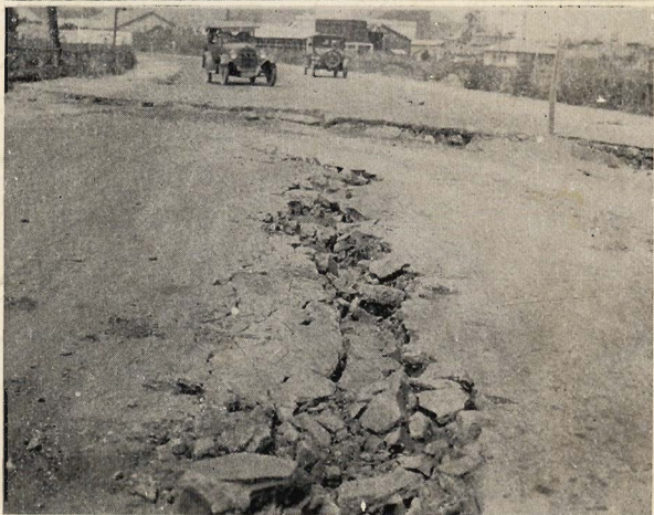
SHEFFIELD DAM RIVEN BY THE QUAKE THE COAST HIGHWAY JUST EAST OF STATE SHOWING CREVICES MADE BY QUAKE
